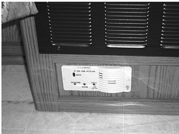
LP Gas Leak Detector
