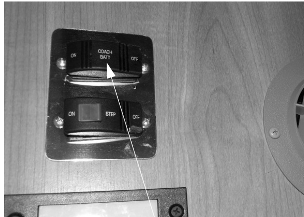
House/Coach Batt Disconnect Switch (Located near entrance door or end of galley, depending on model) -Typical View
