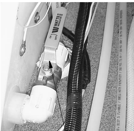
Water Tank Drain Valve (Typical)
