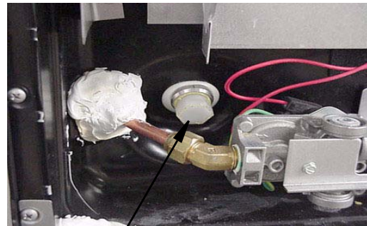
Water Heater Drain Plug Remove with socket
