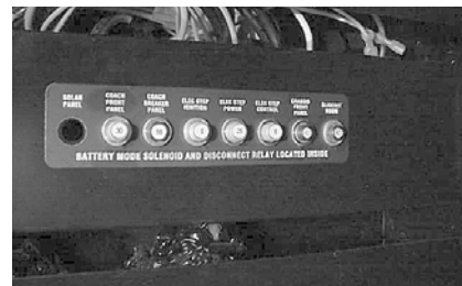
Chassis and House 12V Breakers (cover off)
