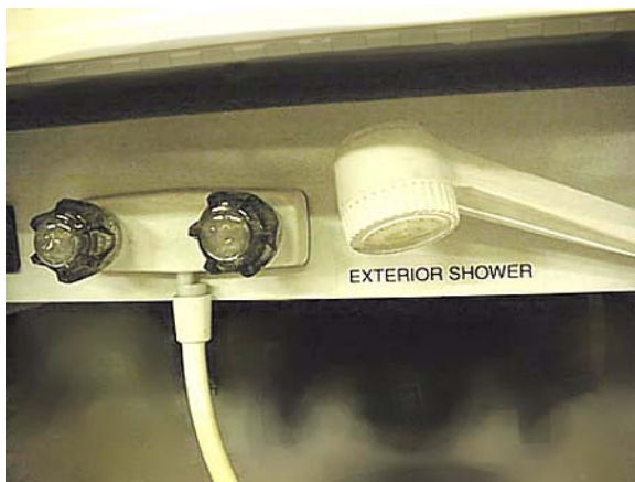
Exterior Shower/Wash Station -Typical View
