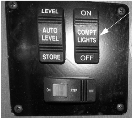
Compartment Lights Switch (Located near entrance door) -Typical View
