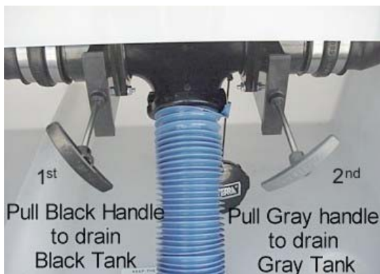
Holding Tank Dump Valves (Typical)
