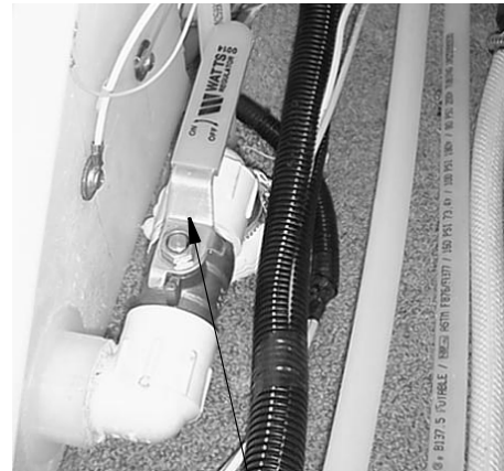
Water Tank Drain Valve (Typical)
