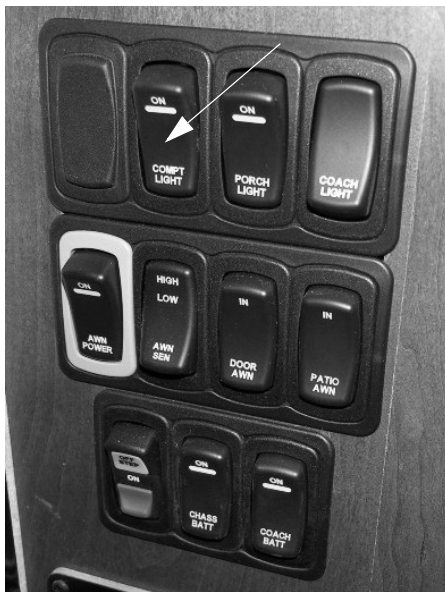
Compartment Lights Switch (Located near entrance door) -Typical View
