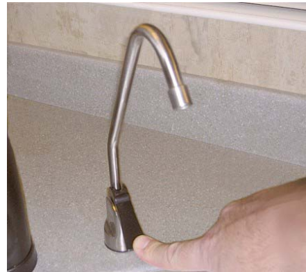
Filtered Water Faucet -Typical View
