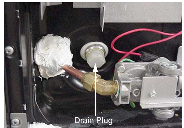
Water Heater Service Access -Typical View
