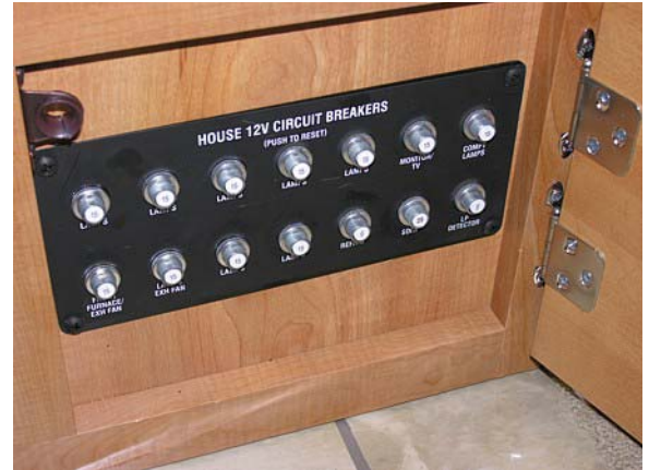
House Circuit Breakers -Typical View
