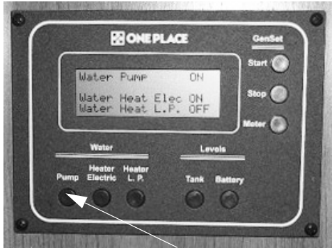
Water Pump Switch
