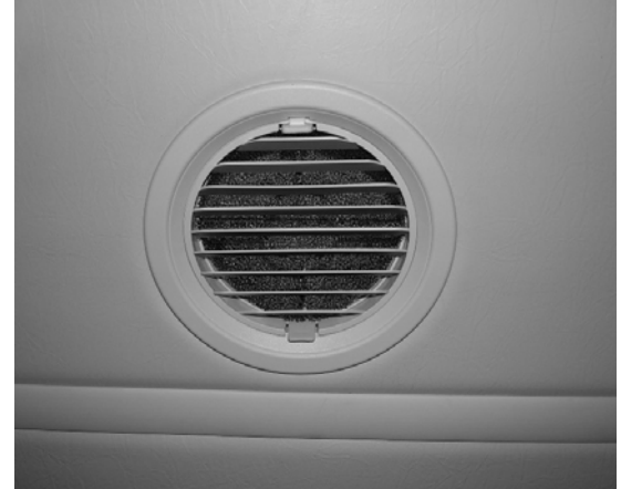
Return Air Vent (Shown with filter installed)
