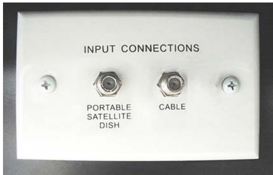
Exterior Connection for Satellite Dish and Cable TV (In Utility Compartment)
