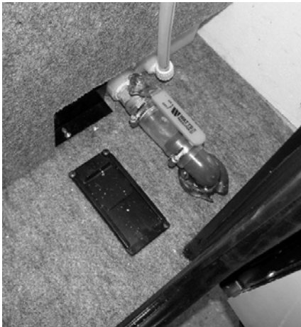
Water Tank Drain Valve (Located in first passenger side compartment) -Typical View
