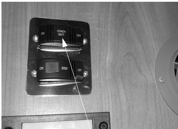
House/Coach Battery Disconnect Switch (Located near entrance door or end of galley, depending on model) -Typical View
