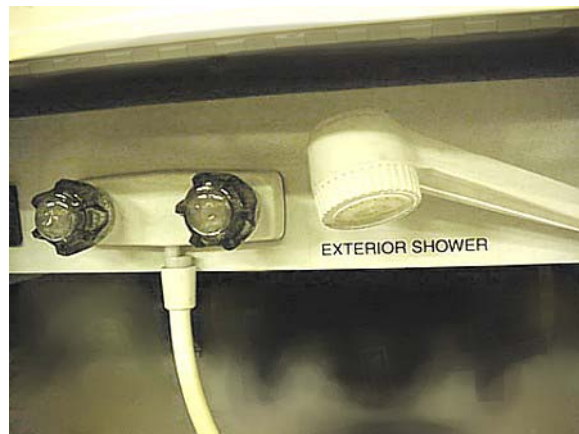
Exterior Shower/Wash Station -Typical View
