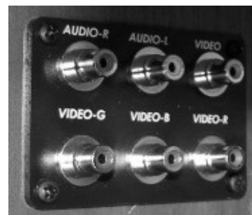
Interior Connection for Satellite Dishes (Located in cabinet near TV)
