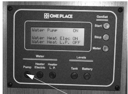
Water Pump Switch
