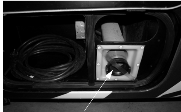
Sewage Drain Hose (Located in utility compartment)
