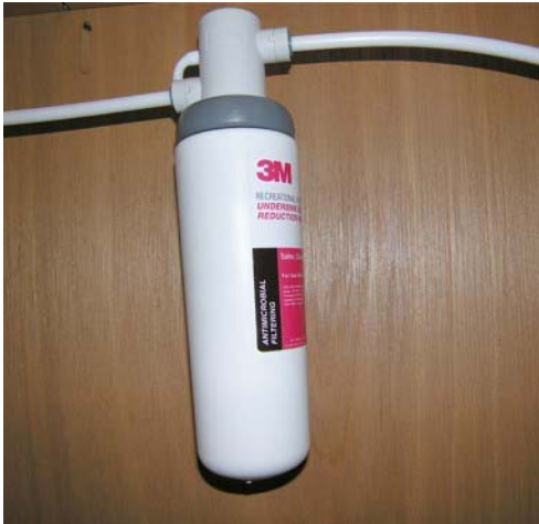
Cold Water Filter Assembly (Located below galley sink) NOTE: Hot waterline is not filtered
