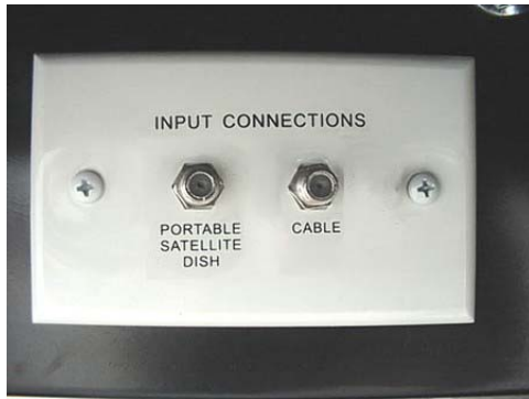
Satellite Dish and Cable TV Input (Hook-up) Connections (Located in utility or service center compartment) -Typical View
