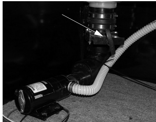
Black Waste Tank Drain Valve #1 (Front) (Located in passenger side compartment ahead of rear axle) -Typical View
