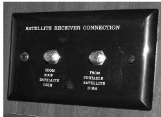
Interior Connection for Satellite Dish (Located in cabinet near TV) -Typical View
