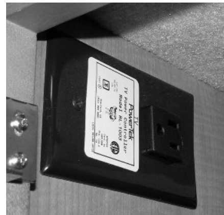
Front TV Ignition Switch Interlock -Typical View
