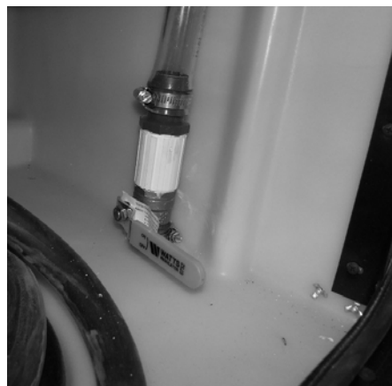
Water Tank Drain Valve (Typical)
