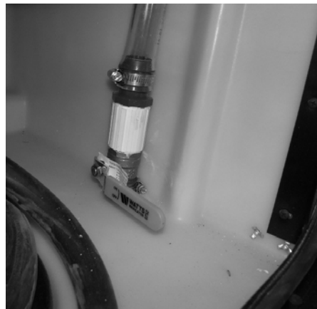
Water Tank Drain Valve (Typical)
