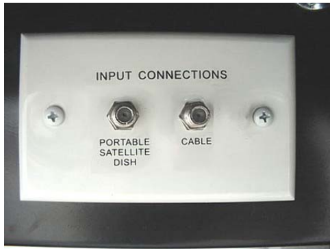
Satellite Dish and Cable TV Input (Hook-up) Connections (Located in utility or service center compartment) -Typical View
