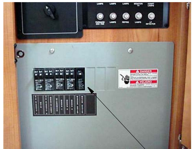
120-Volt House Circuit Breakers -Typical View
