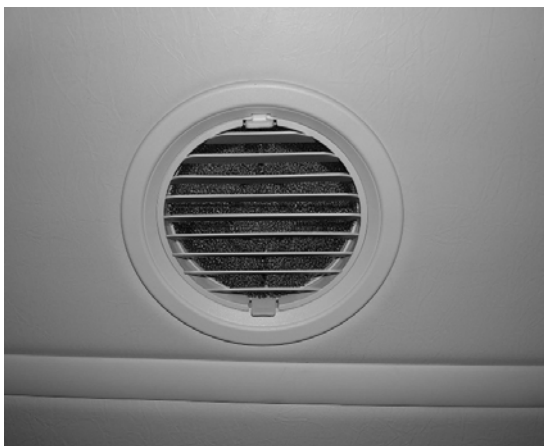
Return Air Vent (Shown with filter installed)
