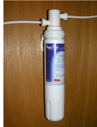
Water Filter Assembly (Located below galley sink) -Typical View
