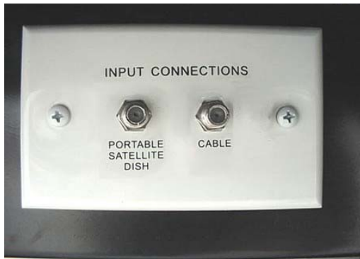
Exterior Connection for Satellite Dish and Cable TV (Located in utility compartment) -Typical View
