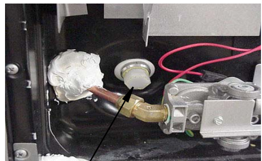
Water Heater Drain Plug (Remove with socket)
