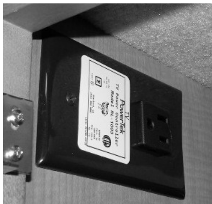
Front TV Ignition Switch Interlock -Typical View
