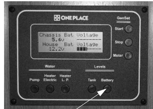
Battery Levels Switch
