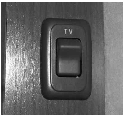
12-Volt Master Power Switch (Located in rear overhead cabinet or on a wall near the TV) -Typical View
