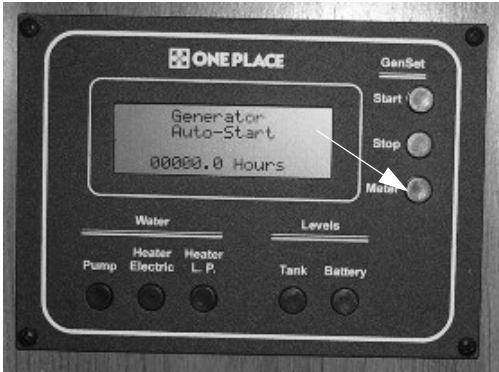
Generator Hourmeter Button -Typical View
