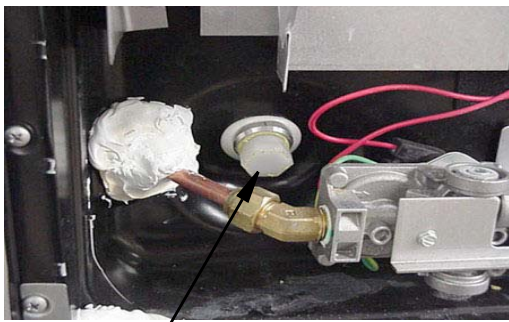
Water Heater Drain Plug (Remove with socket)
