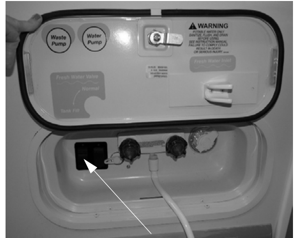
Waste Pump Switch (Located in water service center) -Typical View
