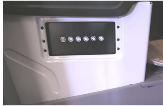
Chassis and House 12V Breakers (Located on side of passenger seat base toward door) * Shown with cover removed -Typical View
