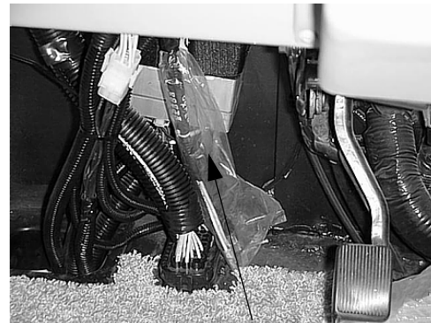
CB Power Wires (in plastic sheath) Typical View - your coach may differ
