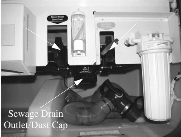
Black and Gray Waste Tank Drain Valves (Located in water service center) -Typical View
