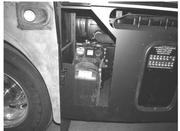
Diesel Exhaust Fluid Fill Tank (Located in passenger or driver side compartment behind rear wheel, depending on model) -Typical View
