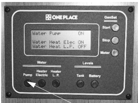
Water Pump Switch
