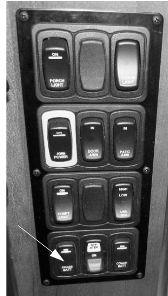
Chassis Battery Disconnect Switch (Located near entrance door) -Typical View
