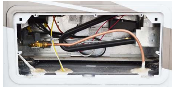
Refrigerator Access Compartment -Typical View
