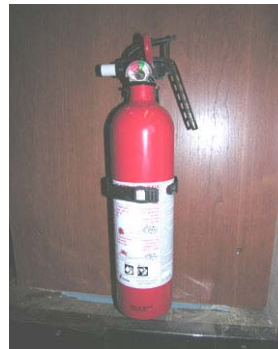
Fire Extinguisher (Typical installation - your coach may vary according to model and floorplan)
