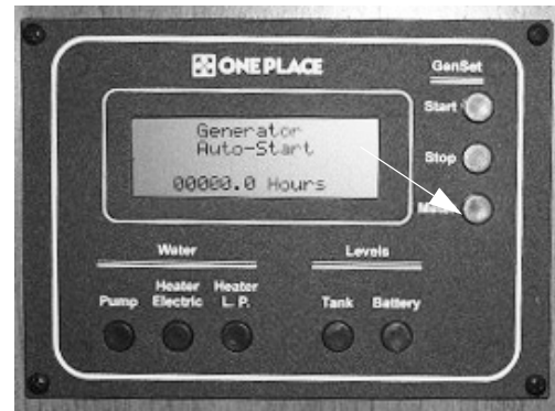
Generator Hourmeter Button -Typical View
