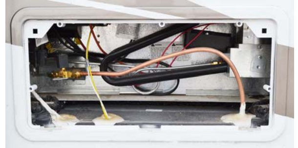
Refrigerator Access Compartment -Typical View
