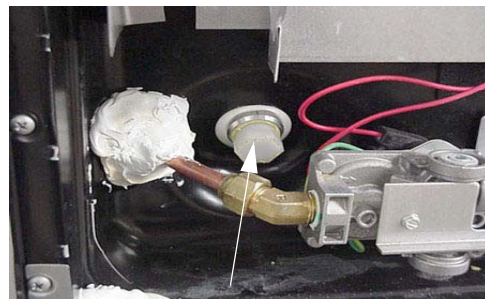
Water Heater Drain Plug (Remove with socket)
