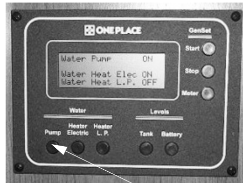
Water Pump Switch
