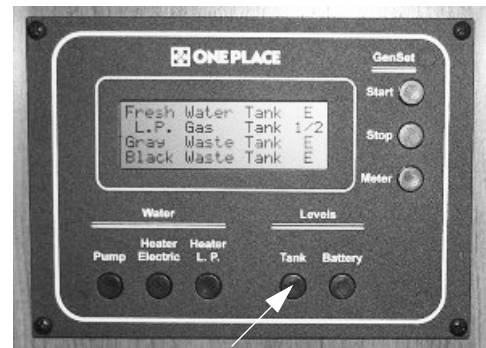
Tank Levels Switch
