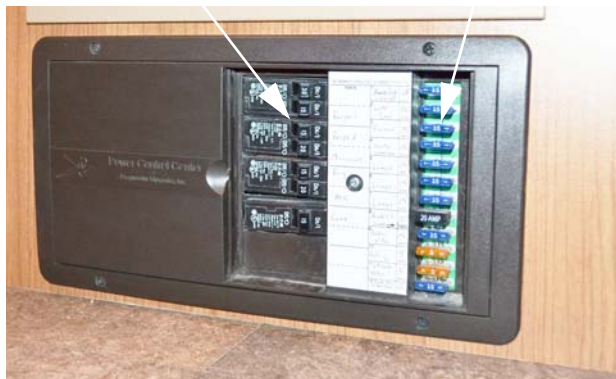
Power Center (Converter) -Typical View
