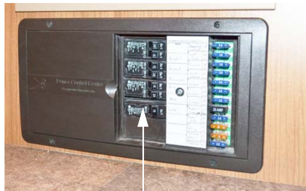
120-Volt Circuit Breakers (Model 70A and 70X) -Typical View
