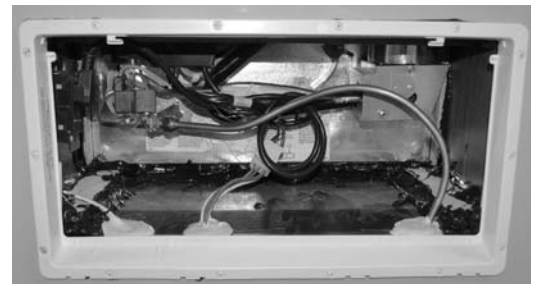
Refrigerator Access Compartment *Shown with cover removed -Typical View
