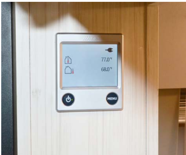
Temperature Control (Located below lounge TV)
