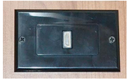
HDMI Connection (Located in cabinet near TV) -Typical View
