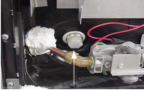
Water Heater Drain Plug (Remove with socket)
