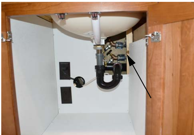
Water Supply Faucets (Located beneath rear bath lavatory cabinet)
