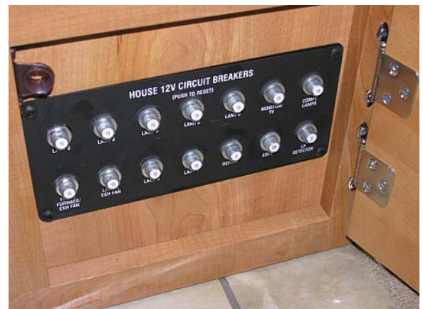
House Circuit Breakers -Typical View
