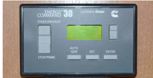
AGS Control Pad (Located near monitor panel)
