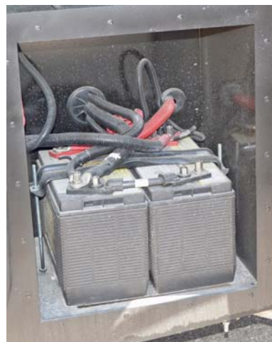
Chassis Batteries (Located behind a rear driver side exterior door) -Typical View
