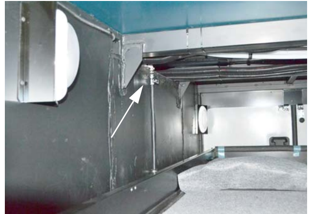
Pot Filler Drain Valve (Located inside middle compartment at front) -Typical View
