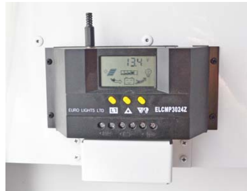
Solar Charge Controller (Located in utility compartment)
