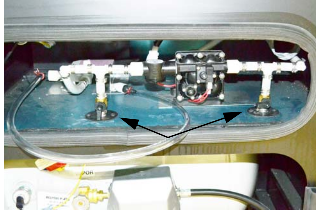
Waterline Drain Valves (Located in driver side compartment) -Typical installation shown
