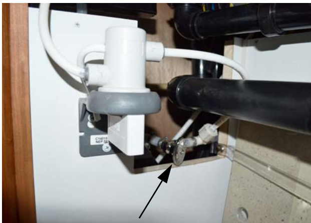
Pot Filler and Ice Maker Water Supply Valve (Located below galley sink) -Typical View
