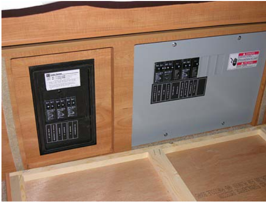
House Circuit Breakers -Typical Installation
