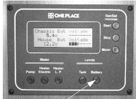
Battery Levels Switch
