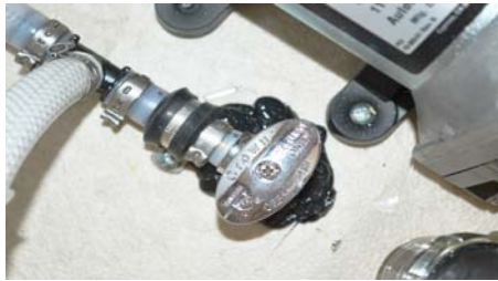
Water Tank Drain Valve (Typical)
