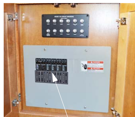
120-Volt House Circuit Breakers -Typical View
