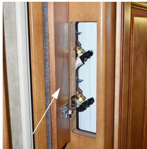
Water Supply Faucets (Located behind access door rear of the washer/dryer cabinet.)
