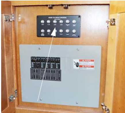
House 12V Breakers -Typical View
