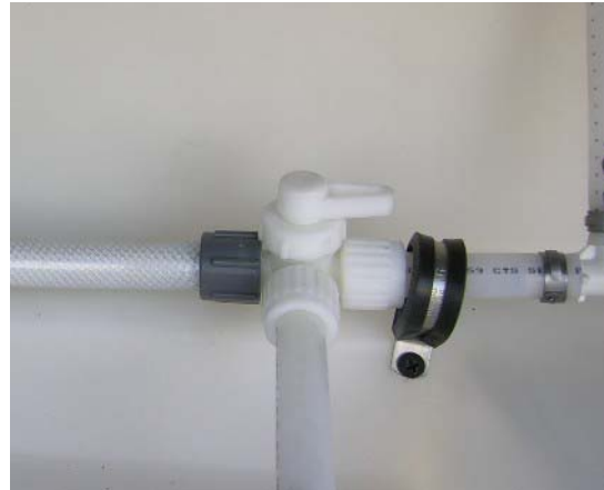
Waterline Drain Valve -Typical installation shown
