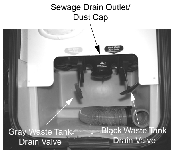
Holding Tank Drain Valves (Located in holding tank compartment) -Typical View
