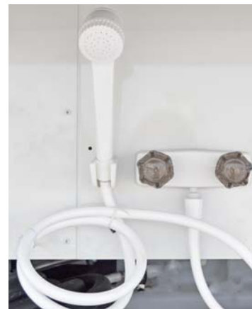
Exterior Shower/Wash Station -Typical View
