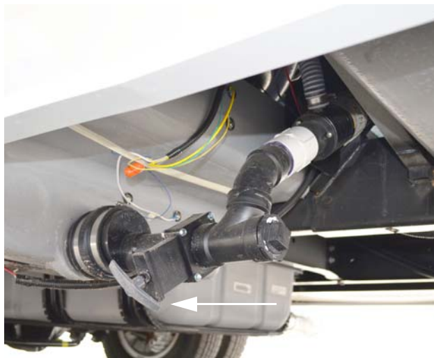
Gray Waste Tank Drain Valve (Located beneath driver side of coach ahead of rear wheel) -Typical View
