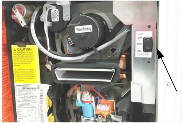
Water Heater Mode Switch (Located behind water heater access panel on exterior of coach)
