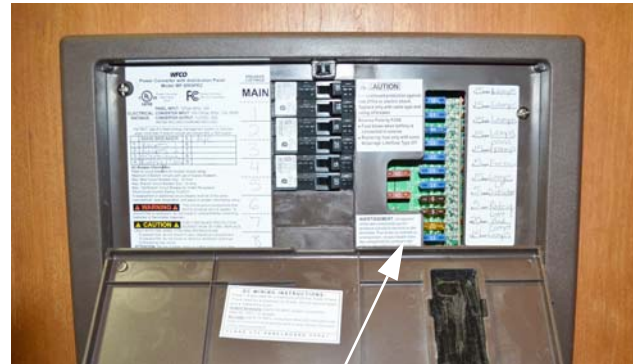
House 12-Volt Fuses (Located on the right-hand side of the power converter) -Typical View
