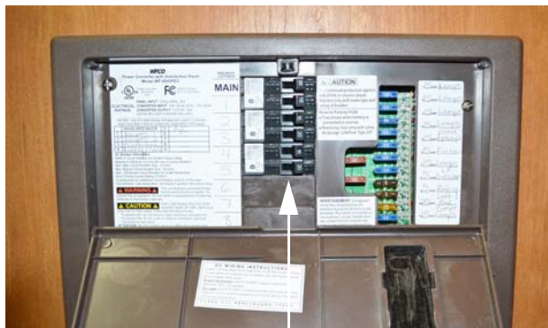
120-Volt Circuit Breakers -Typical View
