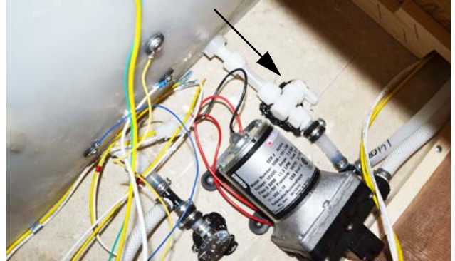
Waterline Drain Valve -Typical View
