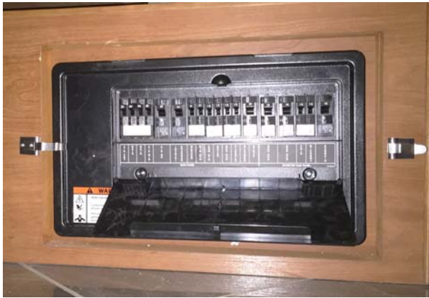
House Circuit Breakers -Typical Installation
