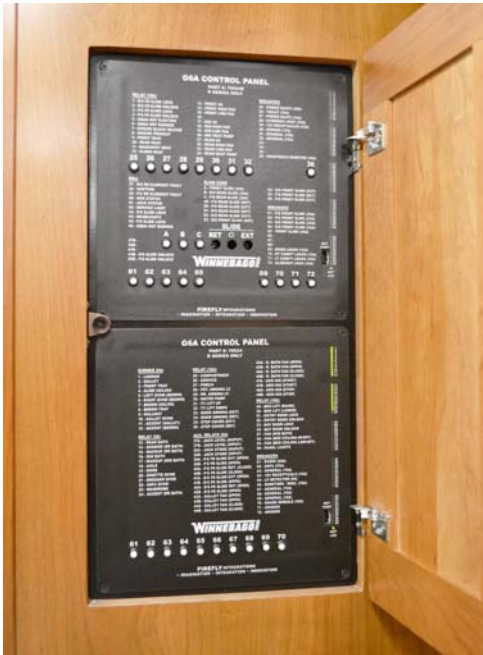
House Circuit Breakers -Typical View
