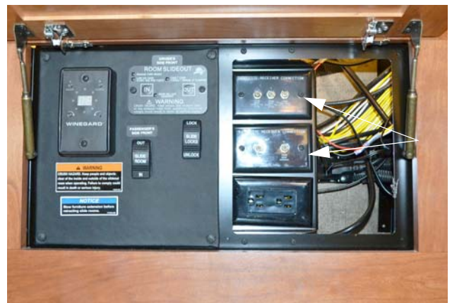
Interior Connections for Satellite Dish (Located in the overhead compartment above entrance door)
