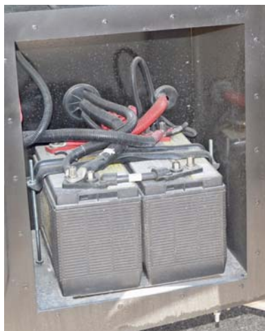
Chassis Batteries (Located behind a rear driver side exterior door) -Typical View
