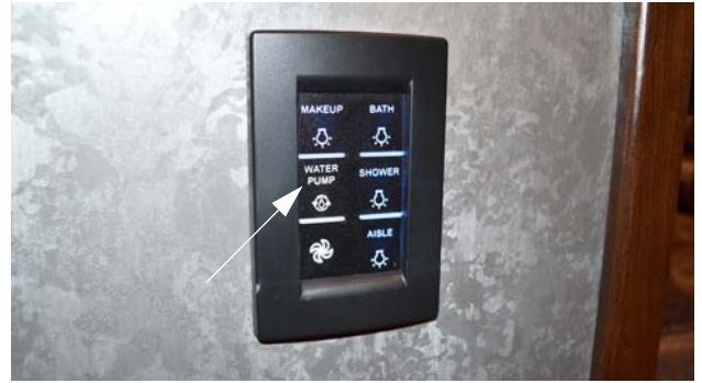
Water Pump Switch (Located in all bath areas) -Typical View The switch will illuminate blue when the switch is on. White illumination indicates the switch is off.
