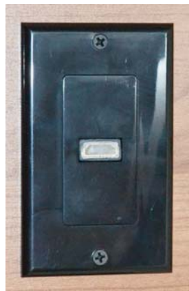
HDMI Connection (Located in a cabinet near TV) -Typical View
