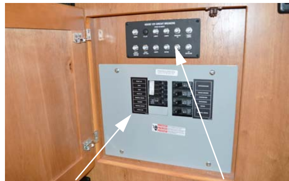
120-Volt Circuit Breakers 12-Volt House Fuses
