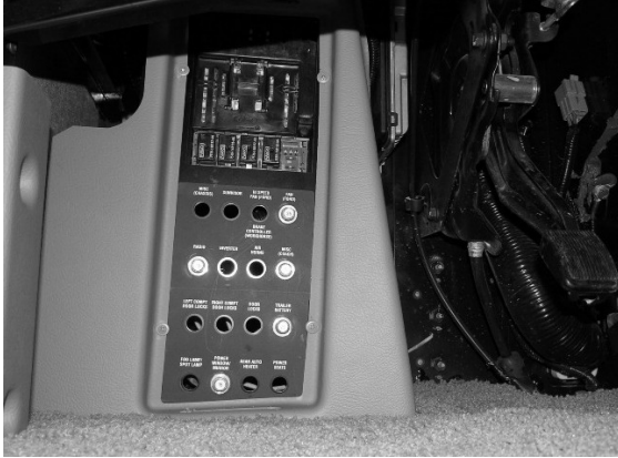
Automotive 12-Volt Circuit Breakers and Fuses (Located beneath left end of dash) -Typical View
