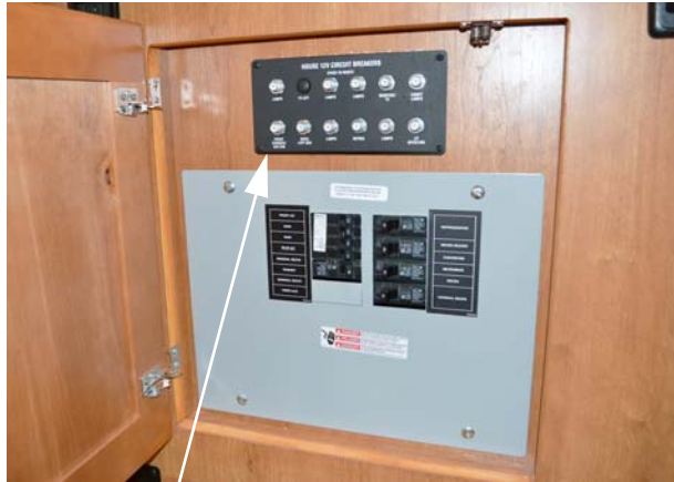
House 12-Volt Circuit Breakers
