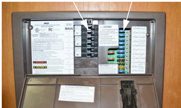
Power Center (Converter) -Typical View
