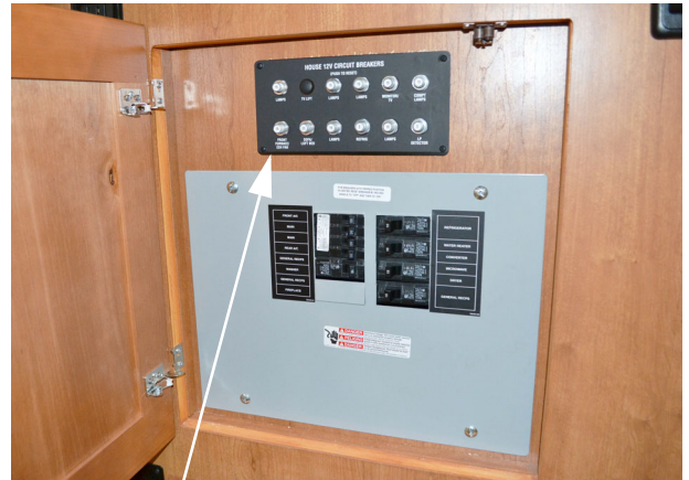
House 12-Volt Circuit Breakers
