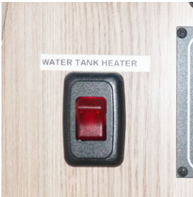
Tank Heater Switch (Located near monitor panel) -Typical View
