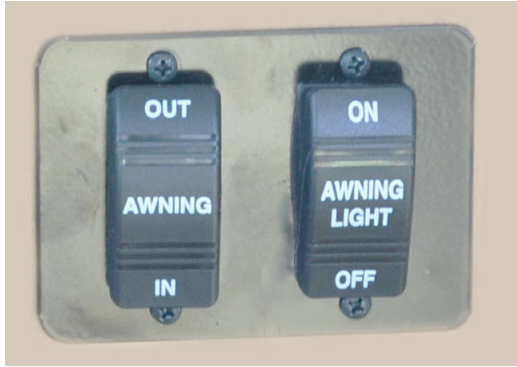
Power Awning Switch and Awning Light Switch (Located at front of galley or shower wall) -Typical View
