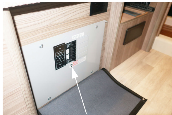
120-Volt Circuit Breakers -Typical View
