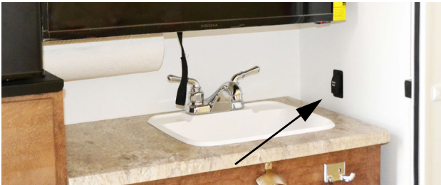
Sink Drain Switch (Located near exterior sink) -Typical View
