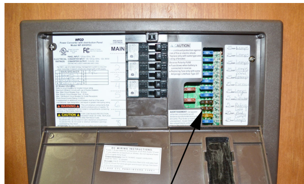
House 12-Volt Fuses (Located on Power Converter) -Typical View
