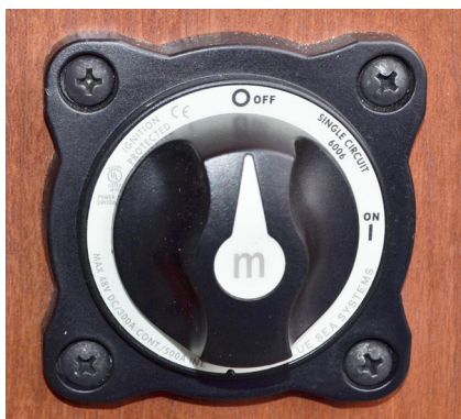
House/Coach Battery Disconnect Switch (Located an exterior compartment near the entrance door) -Typical View
