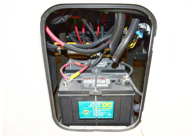
House/Coach Batteries -Typical View
