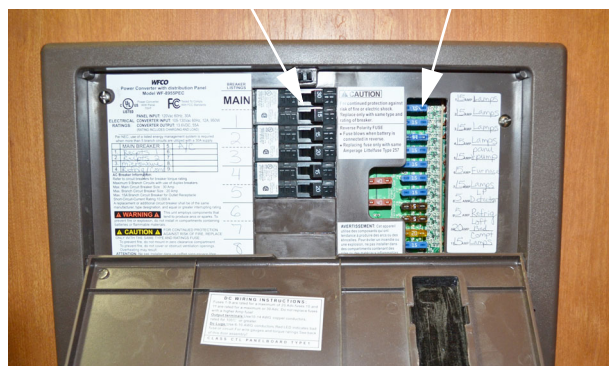
Power Center (Converter) -Typical View
