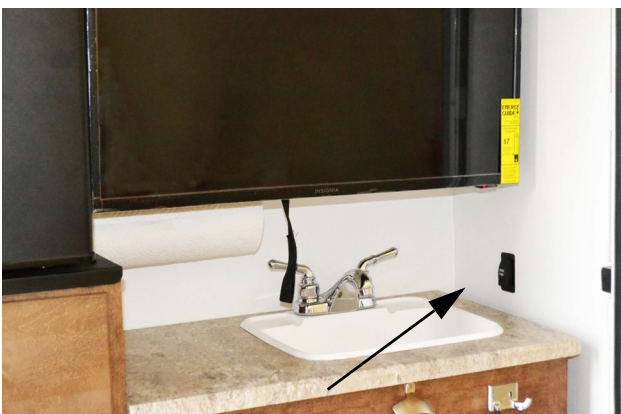
Tailgate Sink Drain Pump Switch (Located near tailgate sink)
