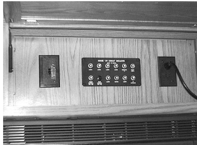
Electric Water Heater Switch above microwave oven
