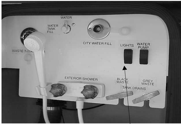
Utility Light Switch
