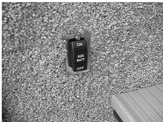
Aux. Batt. Disconnect Switch in Entrance Stepwell
