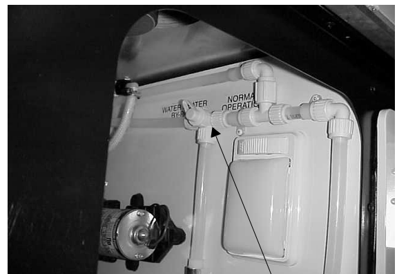
Water Heater Bypass Valve
