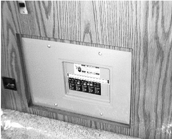
House 110-volt Breaker Panel
