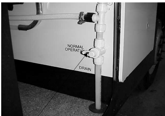
Water Line Drain Valve
