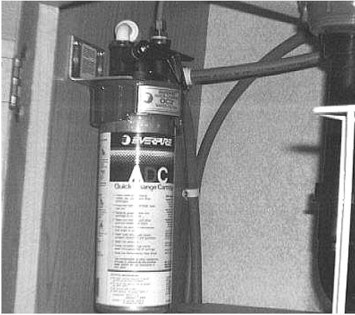
Water Filter Assembly - Below Galley Sink
