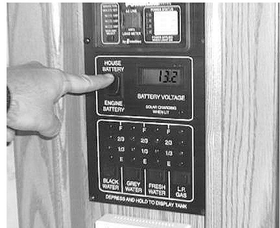
Battery Voltage Check One Place Panel
