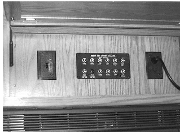
House 12-Volt Breaker Panel
