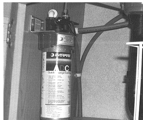
Water Filter Assembly - Below Galley Sink
