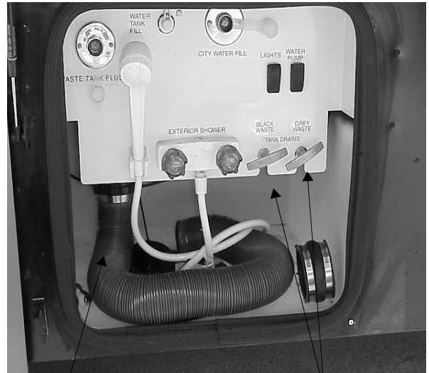
Sewage Dump Outlet & Hose
