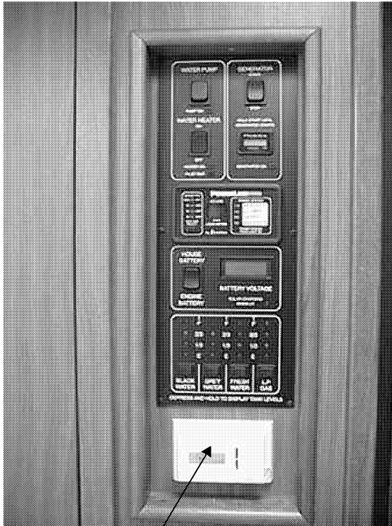
Power Vent Thermostat Bath Area
