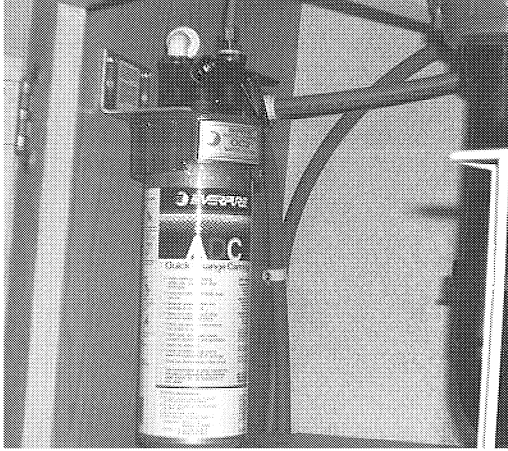
Water Filter Assembly - Below Galley Sink
