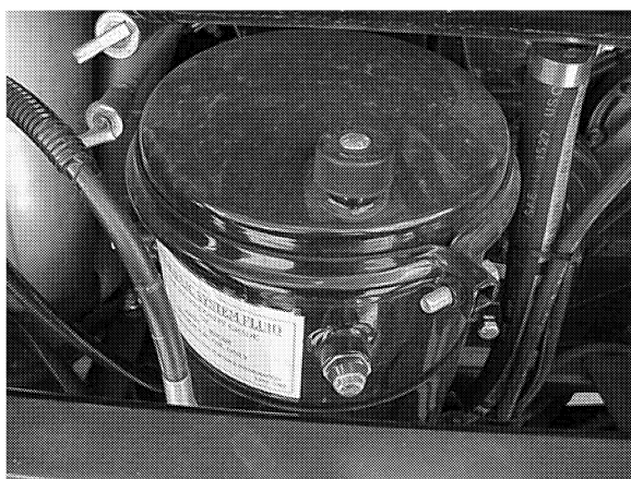
Hydraulic Fluid Tank
