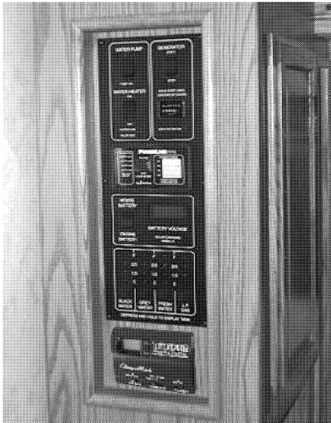
One Place Monitor Panel
