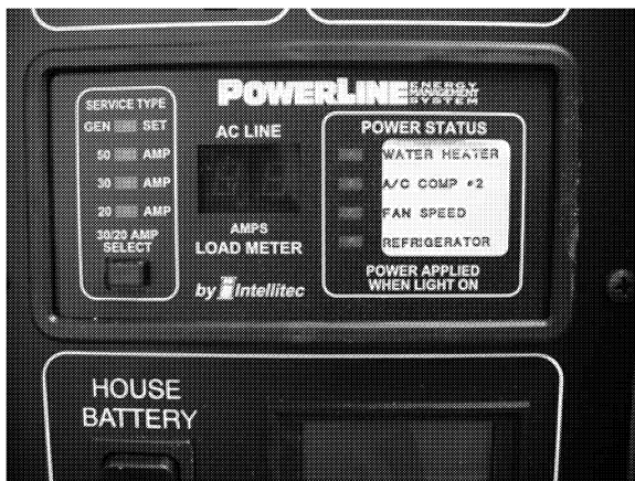
EMS Display on OnePlace Monitor Panel
