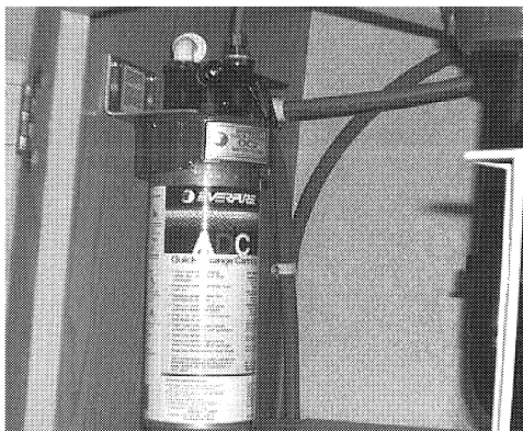
Water Filter Assembly - Below Galley Sink
