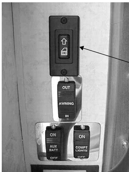
Power Lock Switch (near entry steps)
