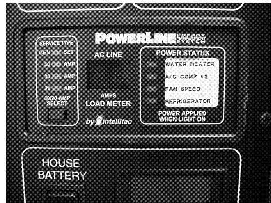
EMS Display on OnePlace Monitor Panel
