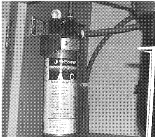
Water Filter Assembly - Below Galley Sink
