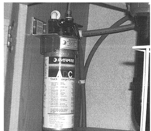
Water Filter Assembly - Below Galley Sink
