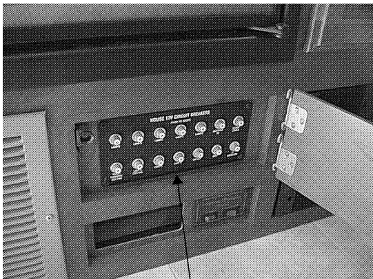
House 12V Breakers
