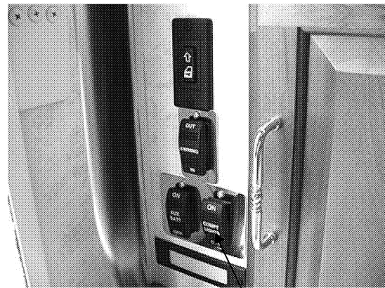
Compartment Lights Switch
