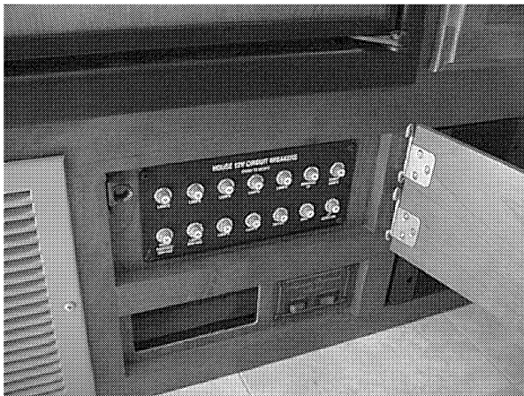
House 12-Volt Breaker Panel
