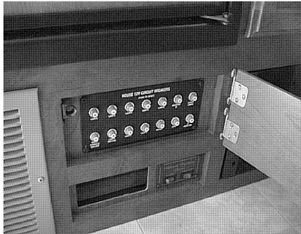
House 12-Volt Breakers
