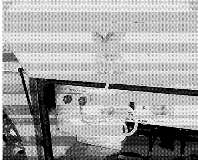
Exterior Shower/Wash Station (Typical)
