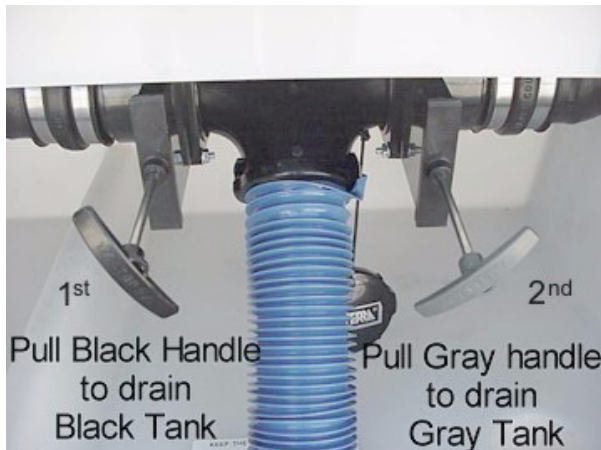
Holding Tank Valves (Typical)
