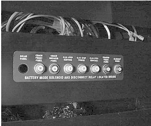
Automotive Fuse/Breaker Panel (Behind Panel on Top Step)
