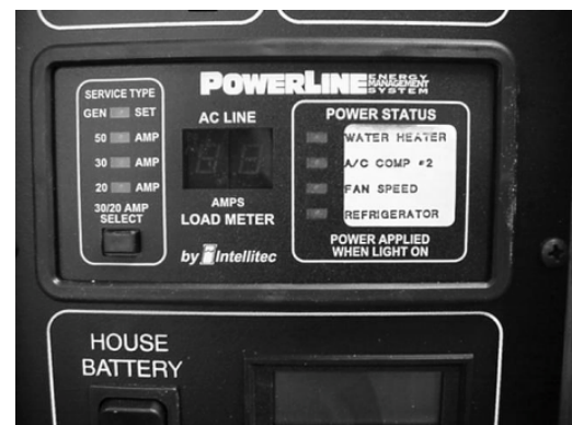
EMS Display on OnePlace Monitor Panel
