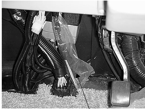
CB Wires (in plastic sheath)
