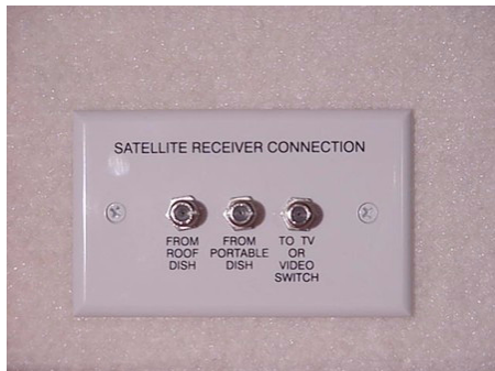
Interior Connection for Satellite Dishes (in front video center cabinet)
