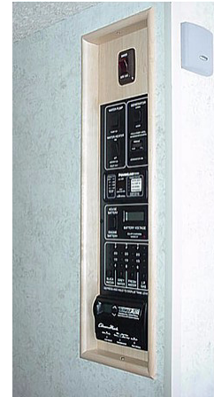
One Place Monitor Panel
