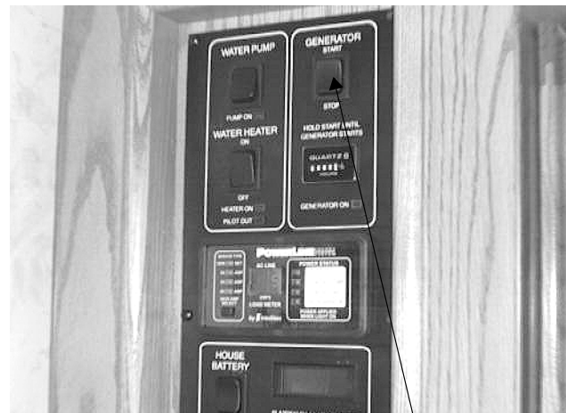
Generator Switch and Hourmeter
