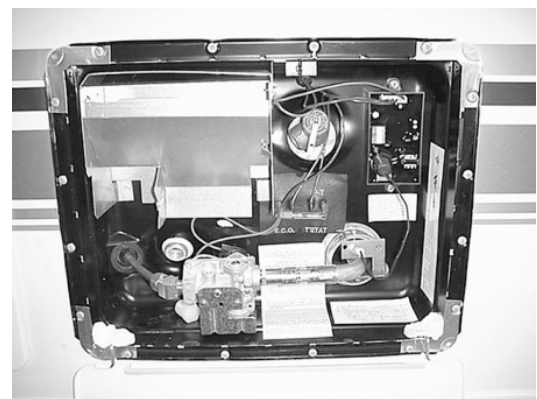
Water Heater Exterior Service Access
