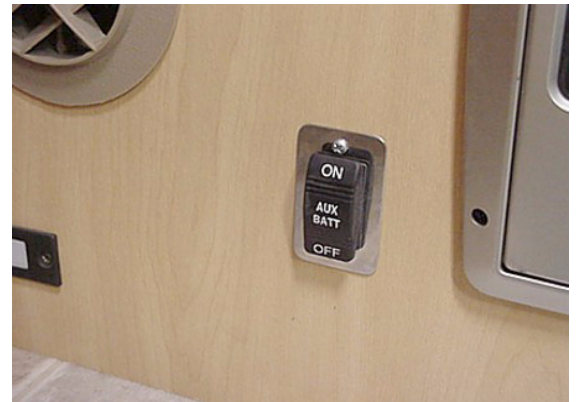
Aux. Batt. Switch (Near entrance door)
