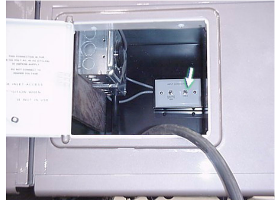
Cable TV Hook-Up in Shoreline Compartment
