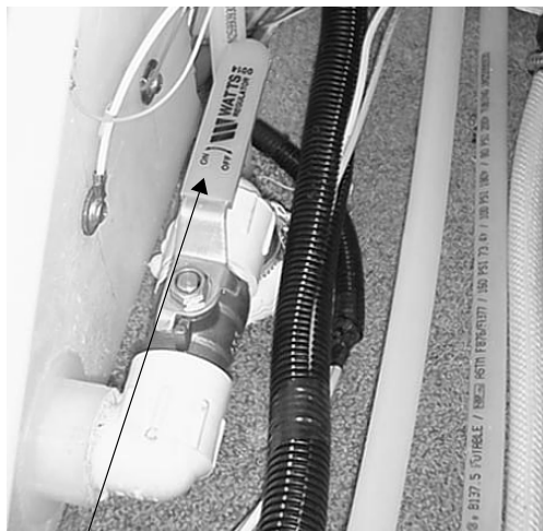
Water Tank Drain Valve
