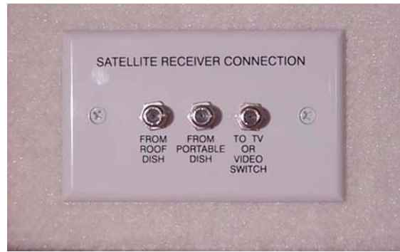
Interior Connection for Satellite Dishes (in front video center cabinet)
