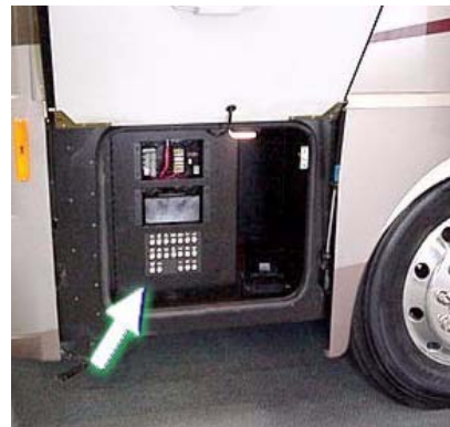
12V Electrical Compartment
