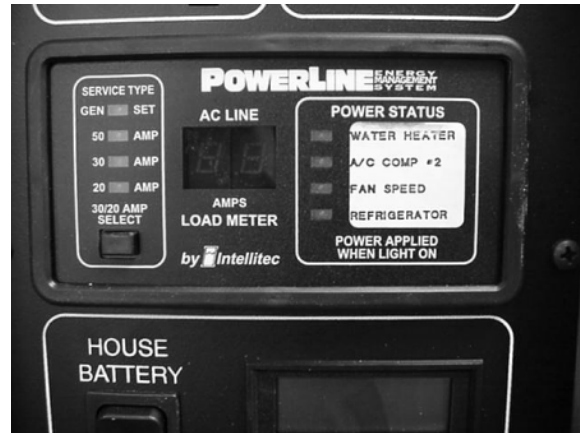
PowerLine EMS Display on OnePlace Monitor Panel
