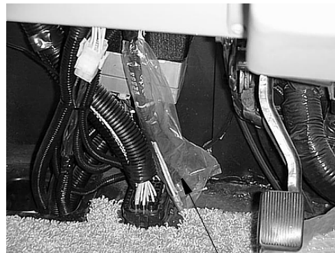
CB Wires (in plastic sheath)
