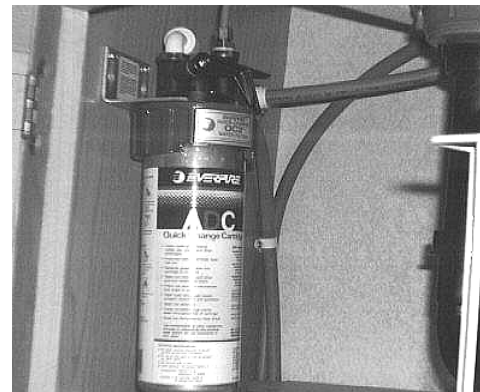
Water Filter Assembly below Galley Sink
