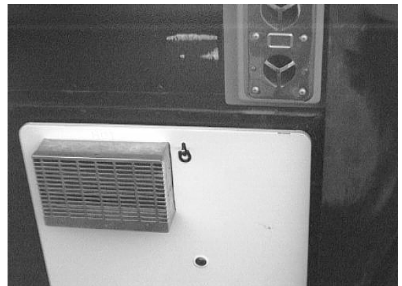
Water Heater Exterior Service Access
