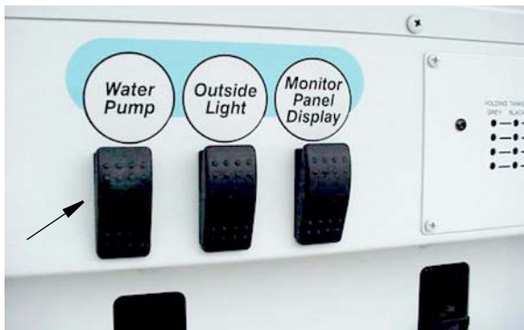
Water Pump Switch in Water Service Center
