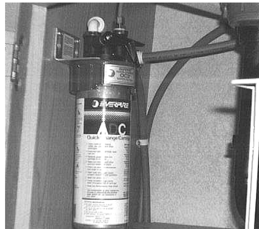
Water Filter Assembly below galley sink
