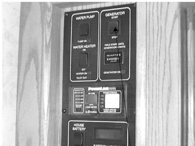
Generator Switch and Hourmeter
