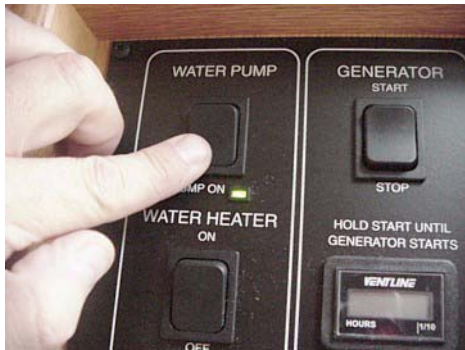
Water Pump Switch on OnePlace Panel
