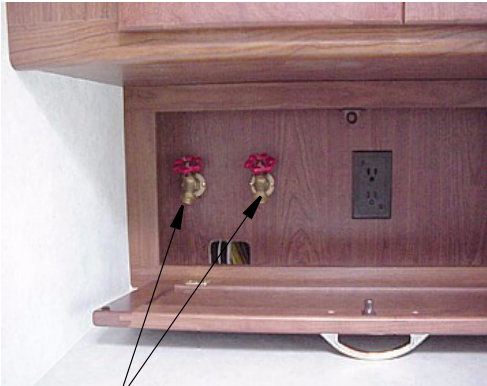
Water Supply Faucets -typical
