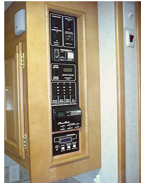
One Place Monitor Panel
