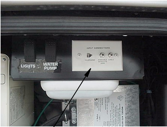
Exterior Input Connections for Satellite Dish, Cable TV and Phone (in Water Center or Shoreline Compartment)
