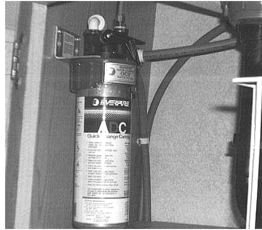
Water Filter Assembly below galley sink
