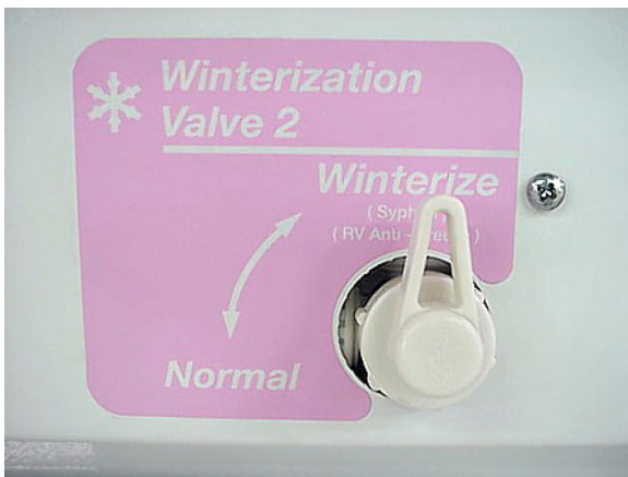
Winterization Valve in water service center
