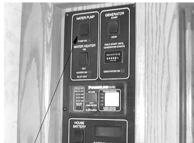
Water Pump Switch
