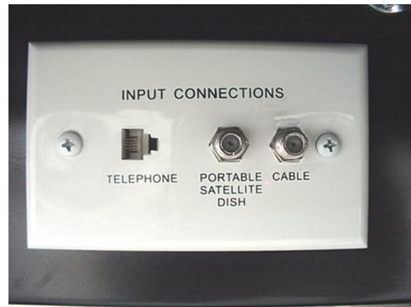
Exterior Connection for Satellite Dishes and Cable TV (In Water Center or Shoreline Compartment)
