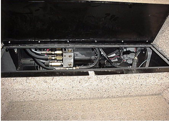
Hydraulic Pump beneath Entry Step
