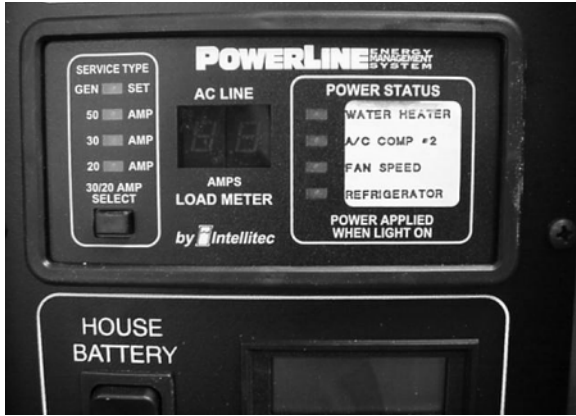
PowerLine EMS Display on OnePlace Monitor Panel
