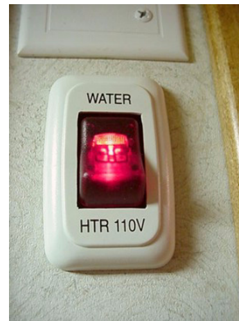
Electric Water Heater Switch (Typical)
