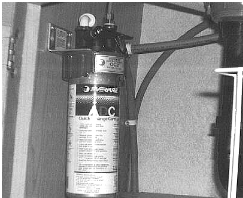
Water Filter Assembly below Galley Sink
