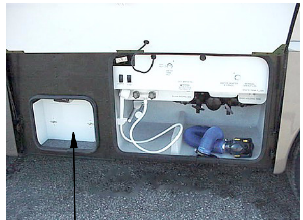
Water drain valves located behind access panel
