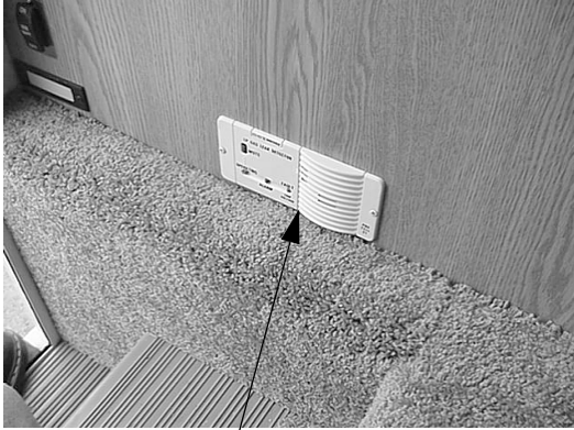
LP Gas Leak Detector
