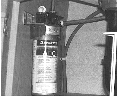
Water Filter Assembly below Galley Sink
