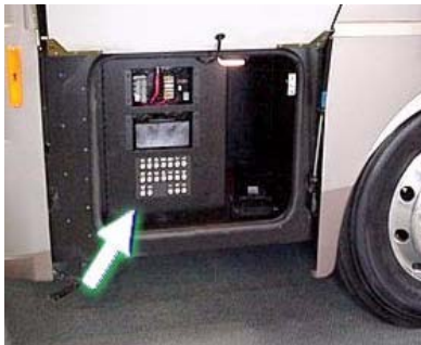
12V Electrical Compartment
