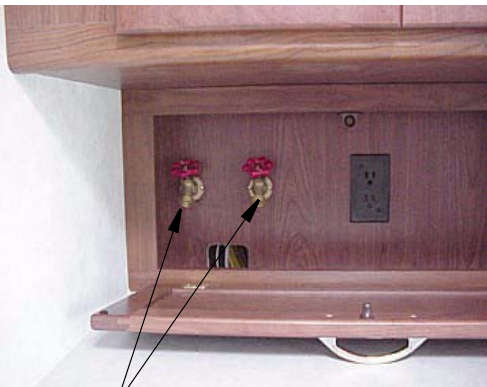
Water Supply Faucets -typical
