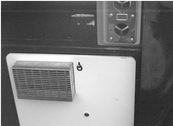
Water Heater Exterior Service Access
