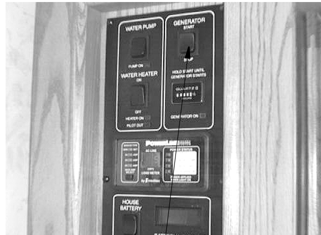
Generator Switch and Hourmeter
