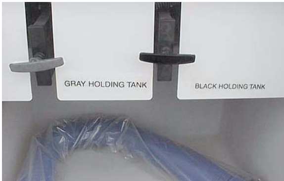
Holding Tank Valves in Water Service Center
