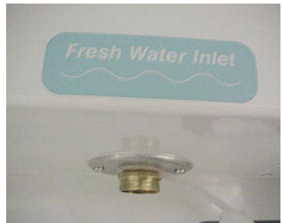
Fresh (City) Water Inlet
