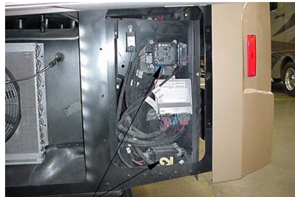
Chassis Fuse & Relay Blocks
