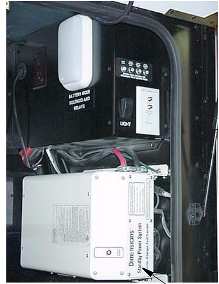
Inverter Charger Unit Location in utility compartment
