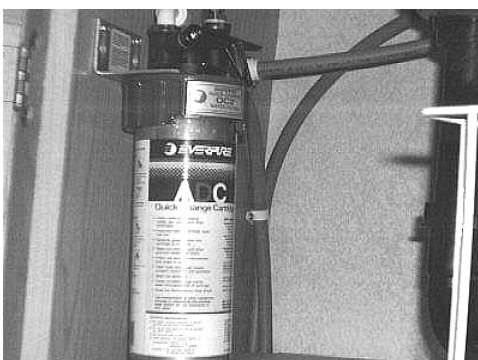
Water Filter Assembly below Galley Sink
