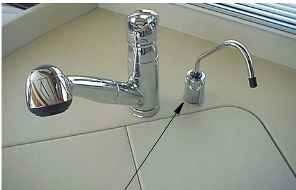
Filtered Water Faucet
