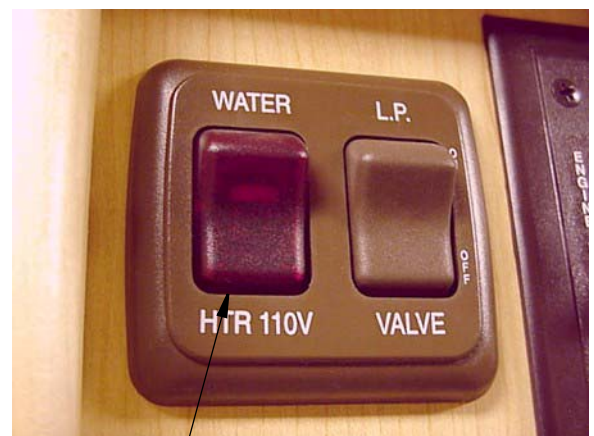
Electric Water Heater Switch (Typical)
