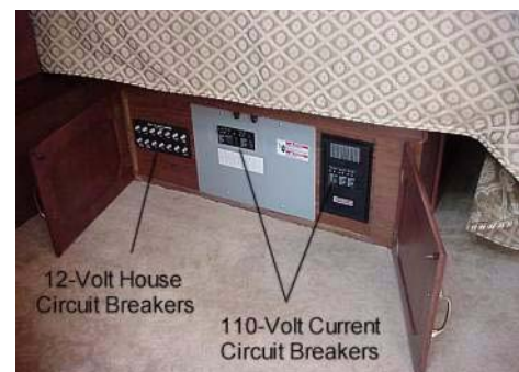
House 12V Breakers
