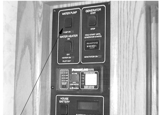
Water Pump Switch
