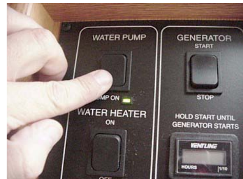
Water Pump Switch on OnePlace Panel
