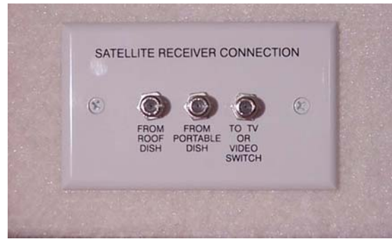
Interior Connection for Satellite Dishes (in front video center cabinet)
