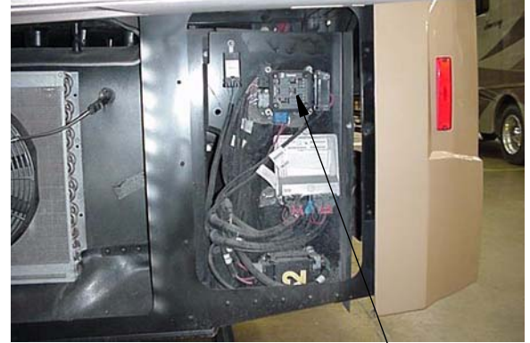
Towing Package fuses are on fuse block
