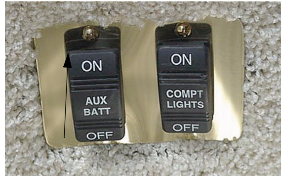
Aux Battery Switch (By Entrance Door)
