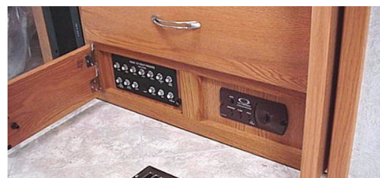
House 12V Breakers (below refrigerator)
