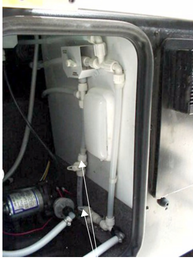
Water Line Drain Valves
