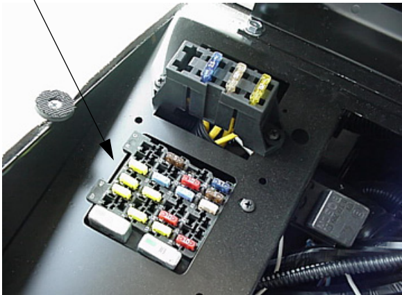
Automotive 12-Volt Fuse Block (Under lift-up dash pod)
