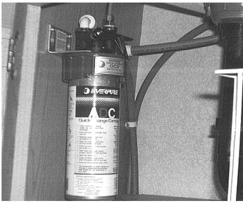
Water Filter Assembly - Below Galley Sink
