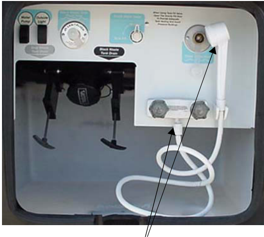
Exterior Shower/Wash Station
