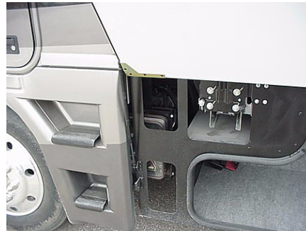
Hydraulic Pump Access - open storage compartment door behind driver's side front tire.
