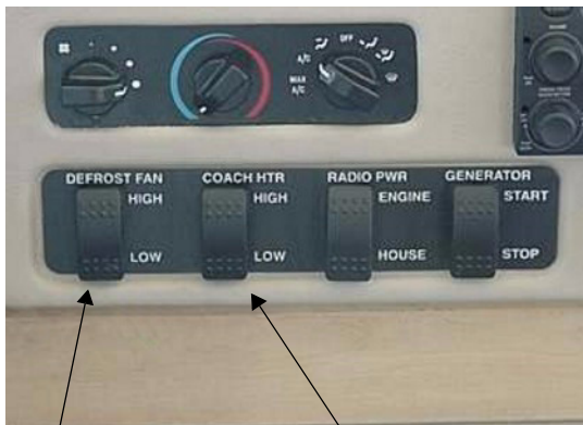
Aux Defrost Fan Switch Coach Heater
