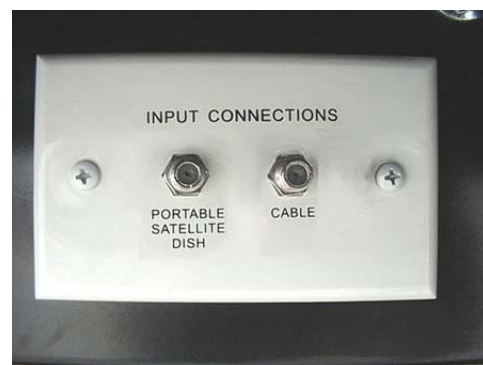
Satellite Dish and Cable TV Input (Hook-up) Connections (in Utility Compartment)
