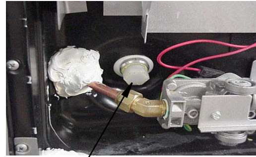
Water Heater Drain Plug Remove with socket
