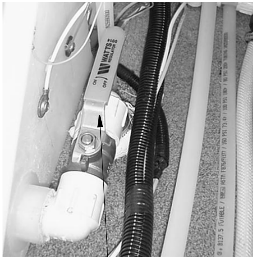
Water Tank Drain Valve (Typical)
