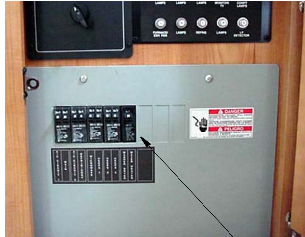
120-Volt House Circuit Breakers
