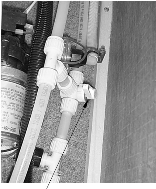
Water Heater Bypass Valve (Typical)
