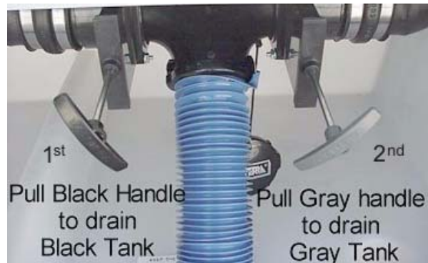
Holding Tank Valves (Typical)
