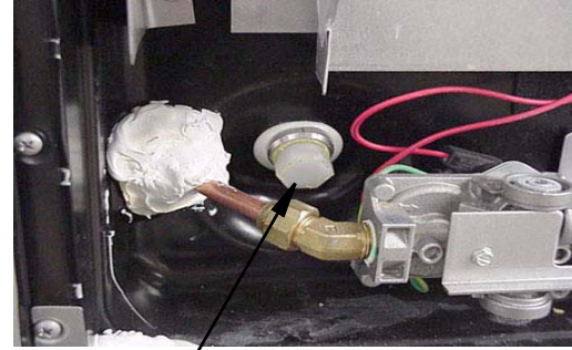
Water Heater Drain Plug (Remove with socket)
