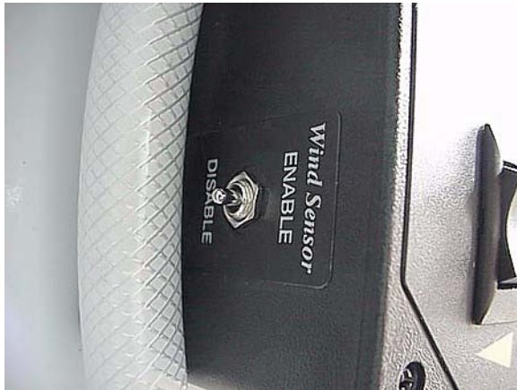
Wind Sensor Control Switch on inboard end of control box.
