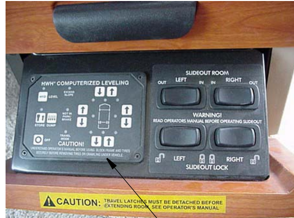
Leveling System Control Panel
