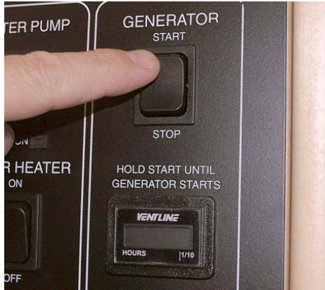
Generator Switch and Hourmeter on monitor panel
