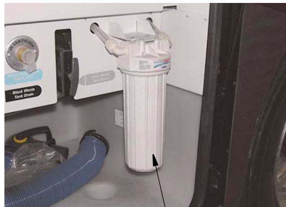
Central Water Filter System in Water Center (typical)
