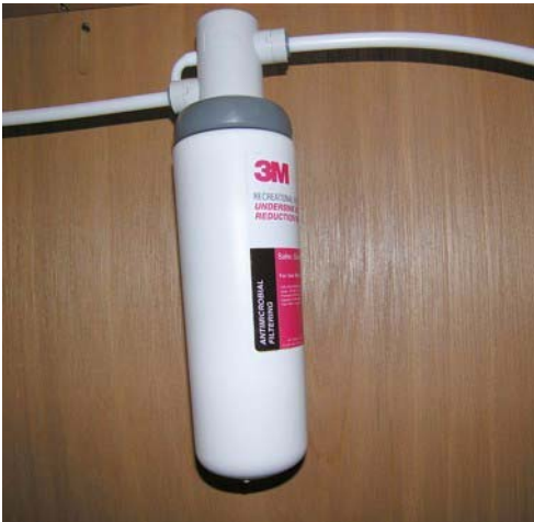
Water Filter Assembly below Galley Sink
