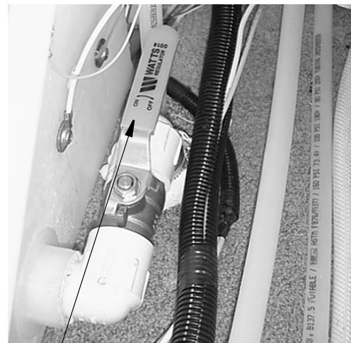
Water Tank Drain Valve
