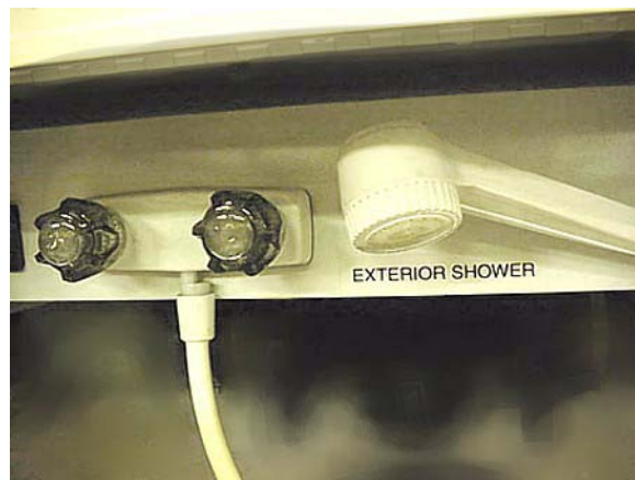
Exterior Shower/Wash Station -Typical View
