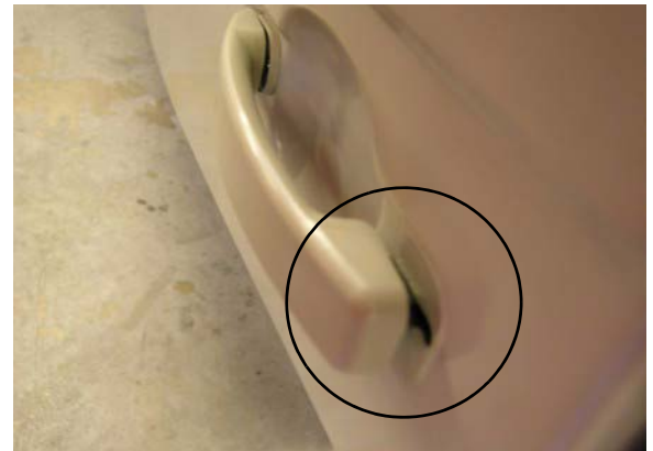
Door Unlatched (note gap)
