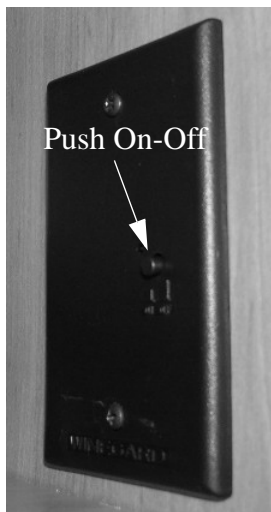
TV Signal Amplifier Power Switch -Typical View
