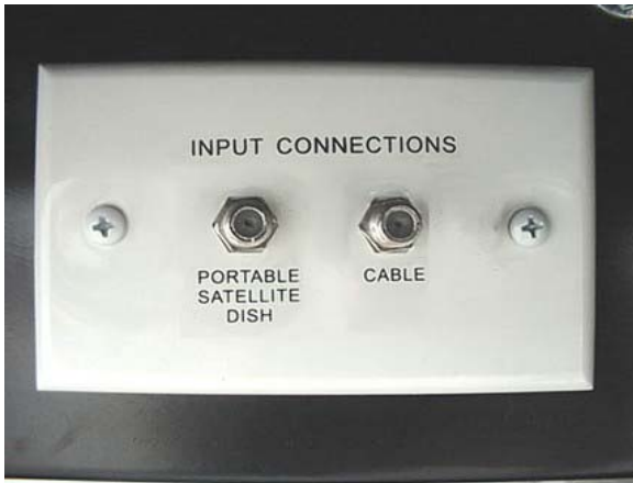
Exterior Connection for Satellite Dish and Cable TV (in the Shoreline Compartment)
