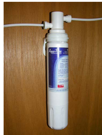
Water Filter Assembly (Located below galley sink)
