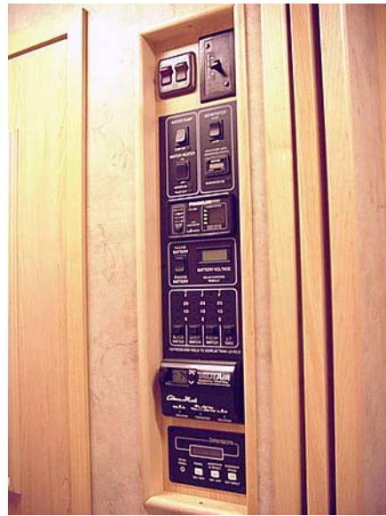
OnePlace Monitor Panel -Typical View
