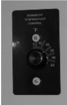
Basement Temperature Control
