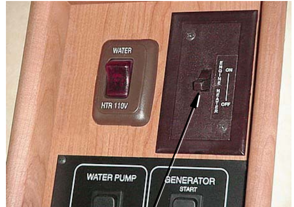
Diesel Engine Heater Switch -Typical View
