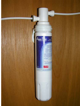
Water Filter Assembly (Located below Galley Sink)
