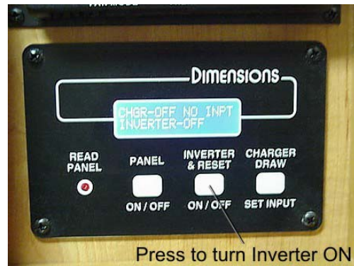
Inverter/Charger Control Panel
