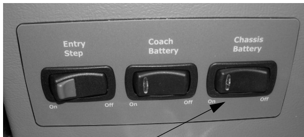
Chassis Battery Disconnect Switch (Located near entrance door) -Typical View
