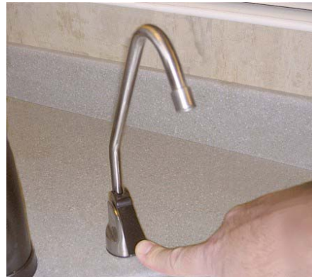
Filtered Water Faucet
