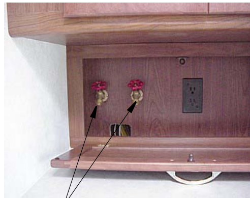
Water Supply Faucets - Typical View
