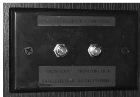
Interior Connection for Satellite Dishes (Located in cabinet near TV) - Typical View
