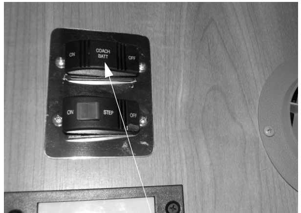
House/Coach Batt Disconnect Switch
