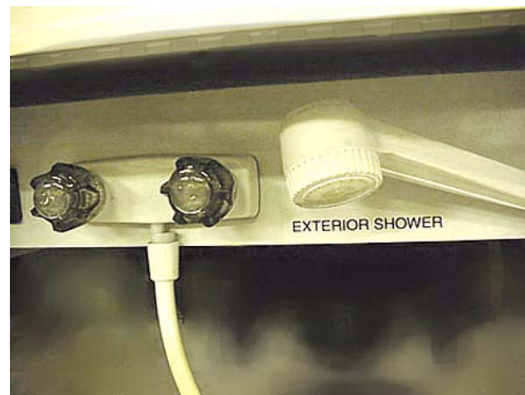
Exterior Shower/Wash Station -Typical View
