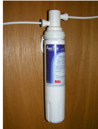
Water Filter Assembly (Located below galley sink)
