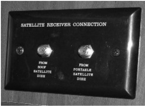
Interior Connection for Satellite Dishes (Located in cabinet near TV) -Typical View
