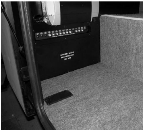
Auto Chassis 12V Circuit Breaker Panel (Located inside passenger side compartment) -Typical View
