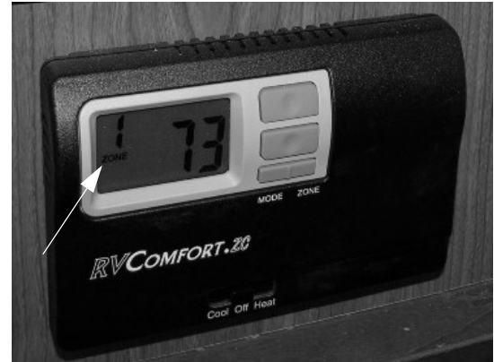
Zone 1 Operation (Living Area/Galley)
