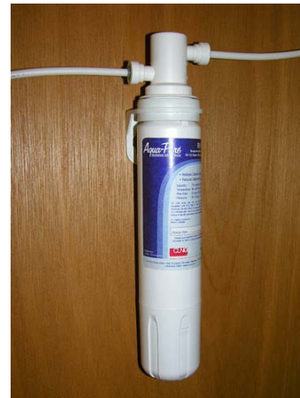
Water Filter Assembly (Located below galley sink)
