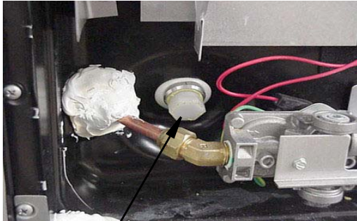
Water Heater Drain Plug (Remove with socket)
