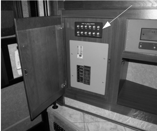
House 12V Circuit Breaker Panel -Typical View
