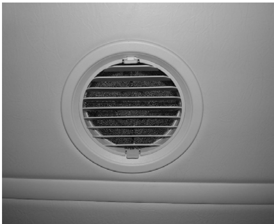
Return Air Vent (Shown with filter installed)
