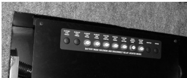
Chassis and House 12V Breakers (Located in passenger side compartment) -Typical View
