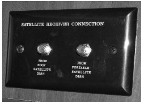
Interior Connection for Satellite Dishes (Located in cabinet near TV)
