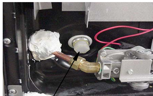
Water Heater Drain Plug (Remove with socket)
