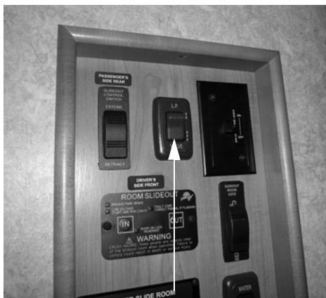
Main Tank Valve Switch (Located near monitor panel area)
