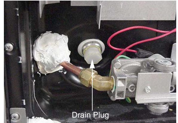
Water Heater Service Access -Typical View
