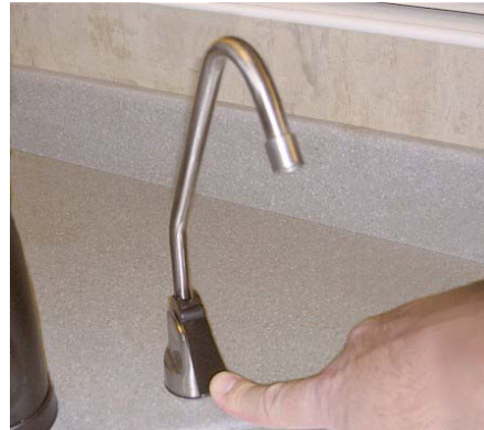
Filtered Water Faucet -Typical View
