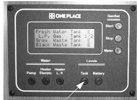
Tank Levels Switch
