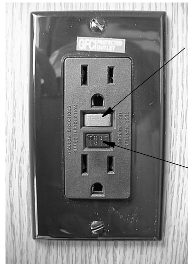
GFCI Outlet (Ground Fault Protector)
