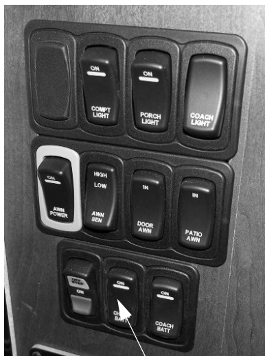
Chassis Battery Disconnect Switch (Located near entrance door) -Typical View
