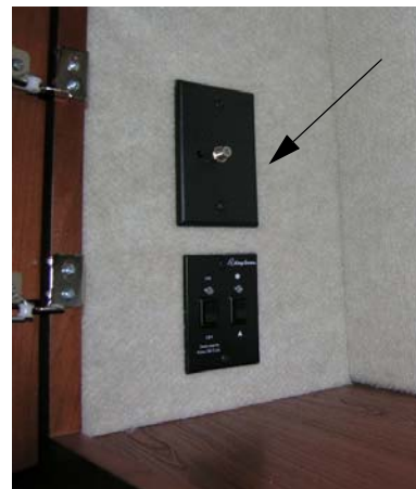
TV Signal Amplifier Power Switch (Located in overhead cabinet above entry door)
