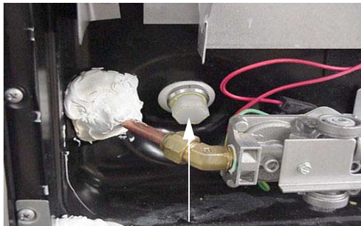
Water Heater Drain Plug (Remove with socket)
