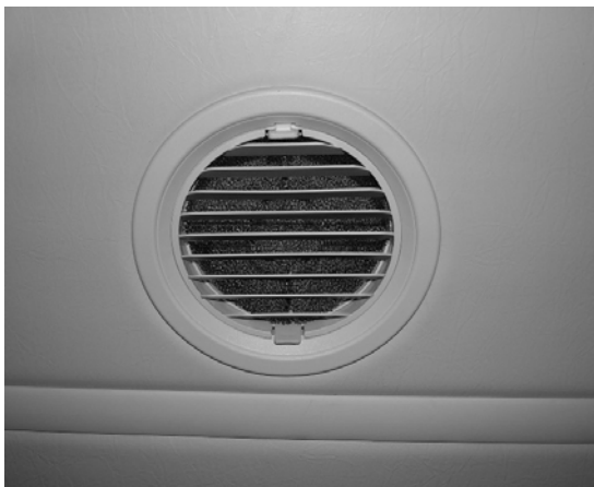
Return Air Vent (Shown with filter installed)
