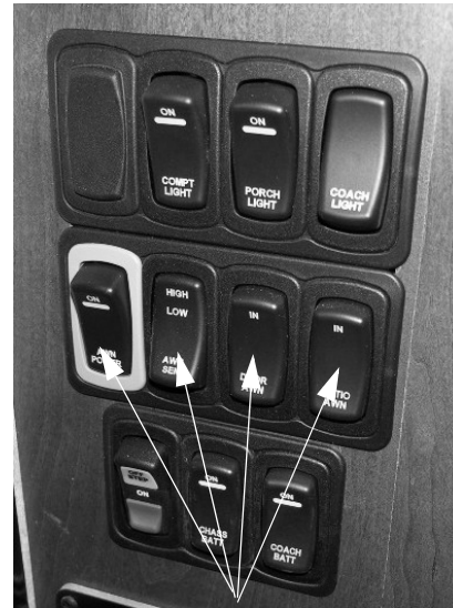
Awning Control Switches (Located near entrance door) -Typical View
