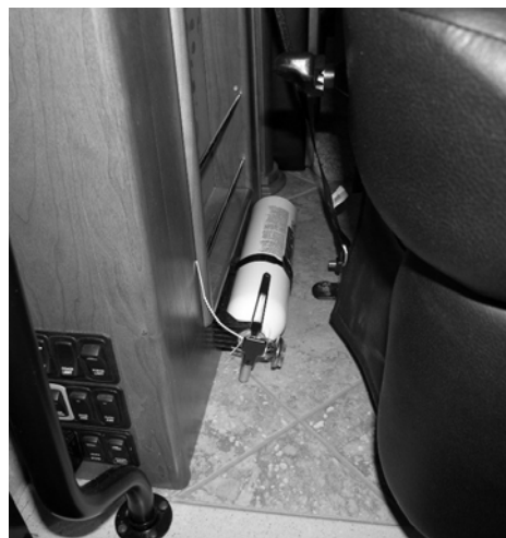
Fire Extinguisher (Located near entrance door) -Typical Installation
