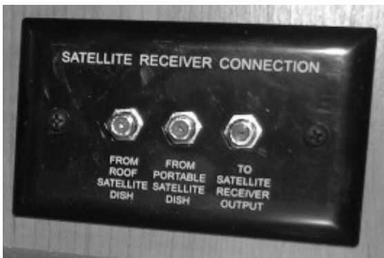
Interior Connection for Satellite Dish (Located near entertainment center cabinet) -Typical View
