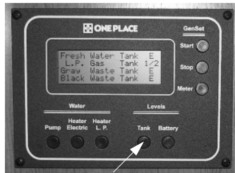
Tank Levels Switch
