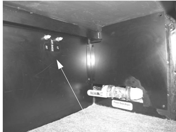
Rear Air Spring Valves (Located in rear driver side compartment)
