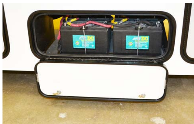
House Batteries (located behind a driver side exterior door) *Model 31C shown
