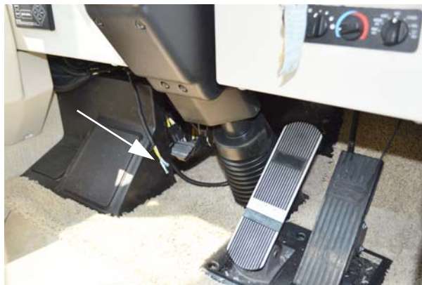
CB Power Wires -Typical View
