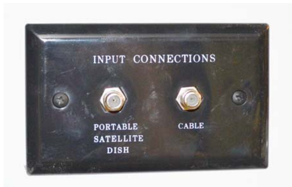
Cable TV and Satellite Dish Connections (Located in utility compartment)
