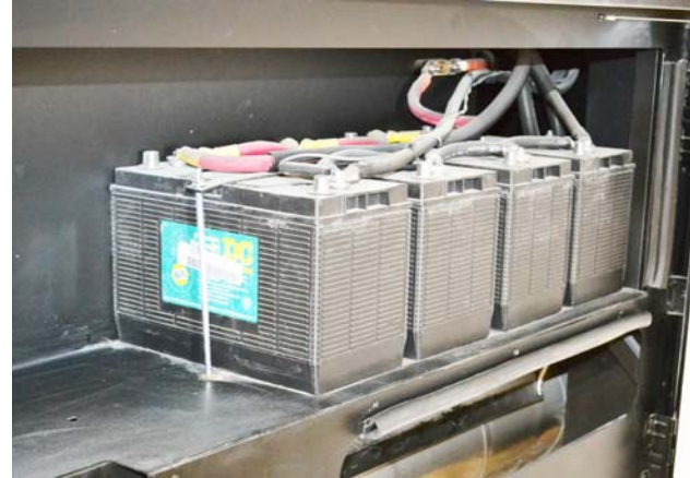
House/Coach Batteries -Typical View
