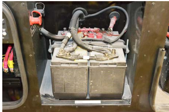
Chassis Batteries -Typical View
