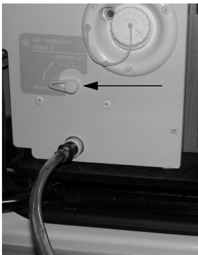
Winterization Valve 2 (Located near the sliding entrance door)
