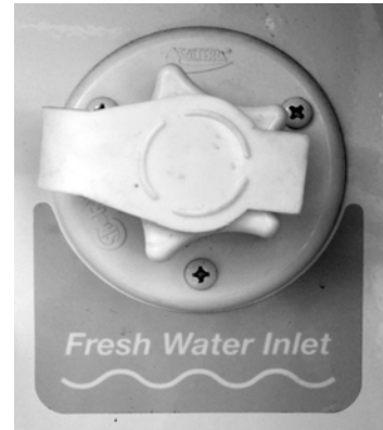
Fresh (City) Water Connection “Fresh Water Inlet” (Located in the water service center)
