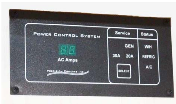
PCS Display Panel (Located near monitor panel) -Typical View
