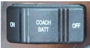
House/Coach Battery Disconnect Switch
