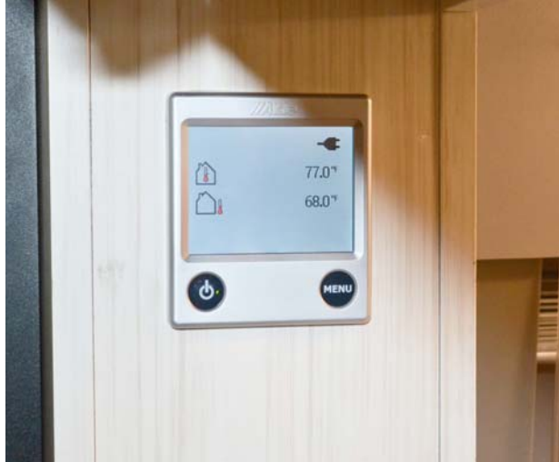
Temperature Control (Located below lounge TV)
