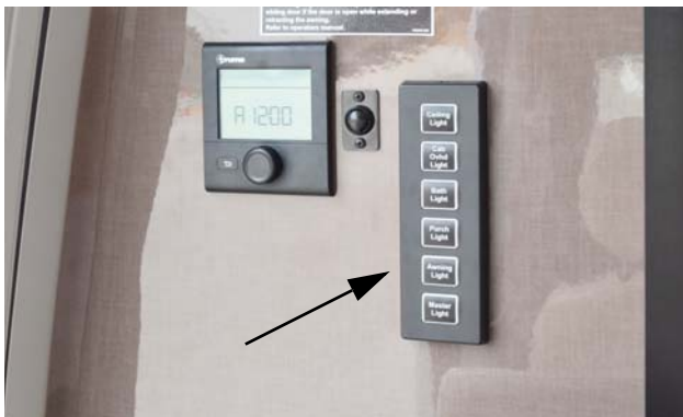
Awning Light Switch (Located near monitor panel or front of galley, depending on model) -Typical View
