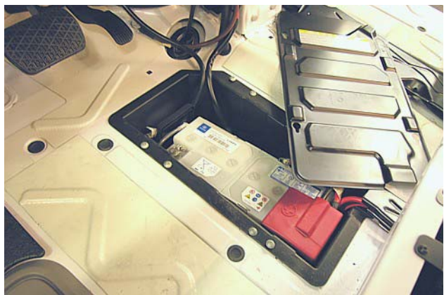
Chassis Battery Access (Located in compartment “well” ahead of driver seat)
