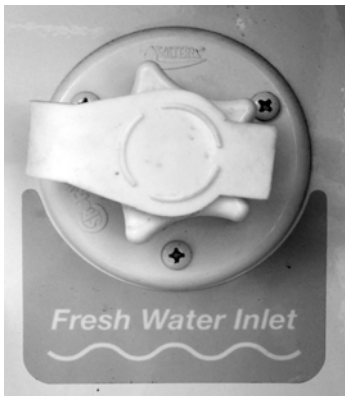
Fresh (City) Water Connection "Fresh Water Inlet"
