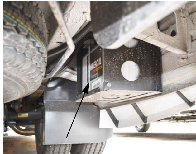
House Battery Access
